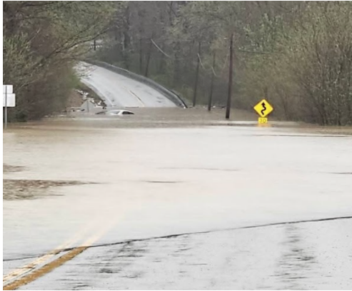
Flooded highways in Nelson County. April, 2025
